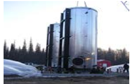
Kenai LNG Plant Produced Water Storage Tanks Provided the secondary containment design for the Injection Well Facility produced water tanks. 2005 to 2006.
