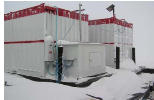
Denali Hotels WWT Expansion Provided three design options for the expansion of the Denali Properties WWT Plant. 2018 to 2019.
