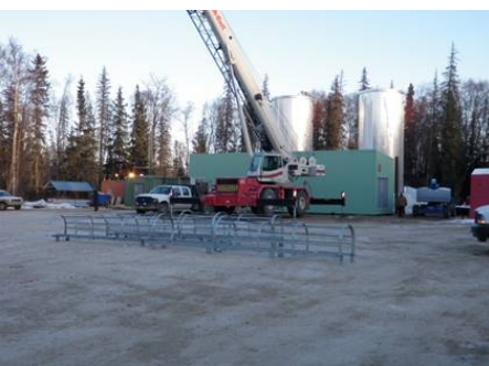
Kodiak WWT Plant. 1998 to 2000. CPAI Water Injection Well System Provided truckable module design for the Beluga River Unit Water Injection Well System. 1992 to 1993.
