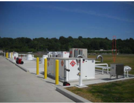
Mente Aviation Fueling System Provided the design for a new state of the art aviation fueling system at the King County Airport. 2015-2017.
