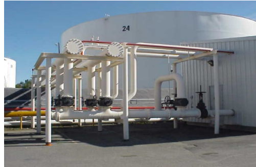
Chevron Bulk Fuel Storage Facility Provided the design for the Chevron Port of Alaska 680,000 tank farm including rail loading. 1997-2011.
